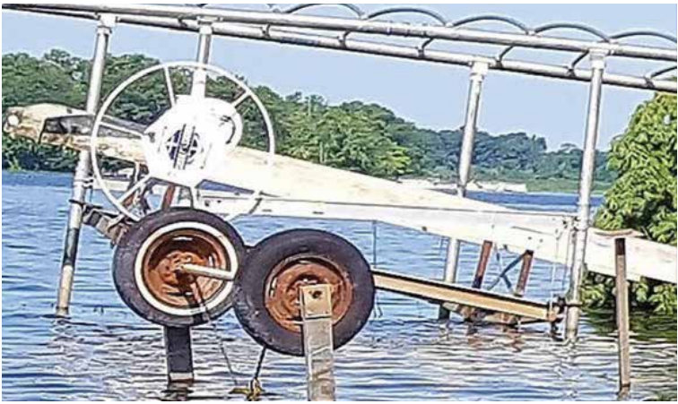
Lifts and docks were looked like broken Tinker Toy models after the storm. Photo by Chuck Knapp
