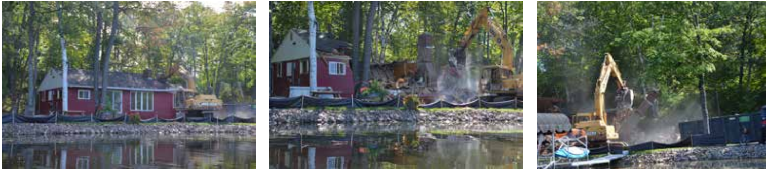
The Walker cabin at the south end of the lake was demolished this fall.
